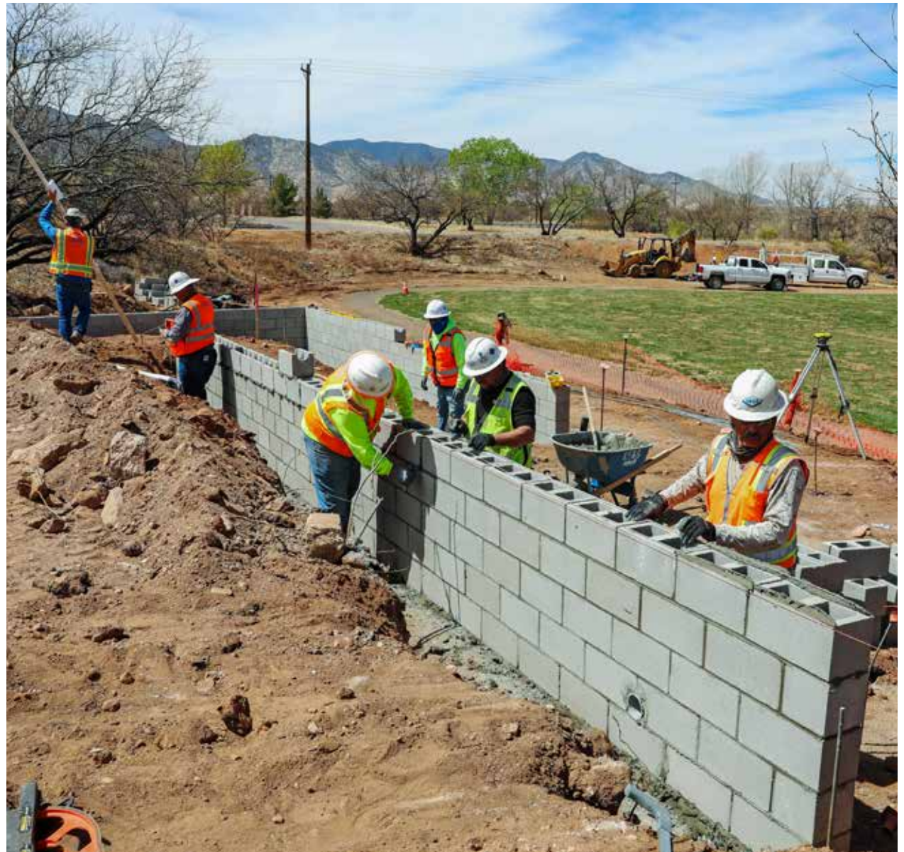
KE&G workers lay blocks as part of City improvements taking place at Soldiers Creek Park and across North Garden Avenue at Landwehr Plaza.
