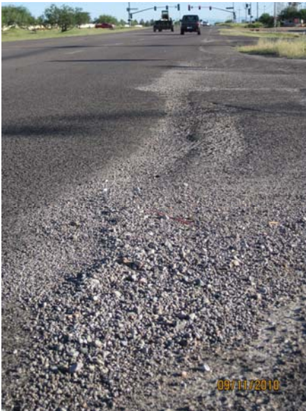
Example of debris and gravel on SR 92. Photo Source: Thomas Armstrong
