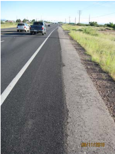
Example of an irregular shoulder on SR 92 that can cause a hazard to bicycle riders Photo Source: Thomas Armstrong
