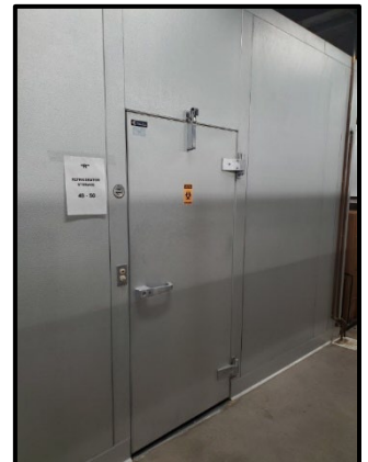
Walk-in freezer storage
