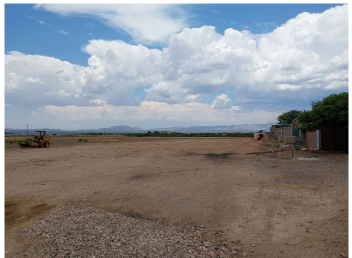
Site prep of land adjacent to the north side of the shelter for expansion
