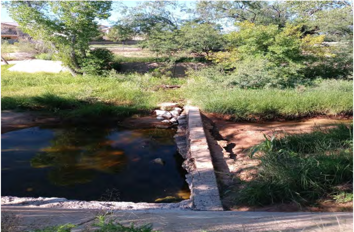
Figure 4.8.4 - 3 rd Street Drainageway about 200-feet upstream of the Woodcutters Canyon Wash Confluence
