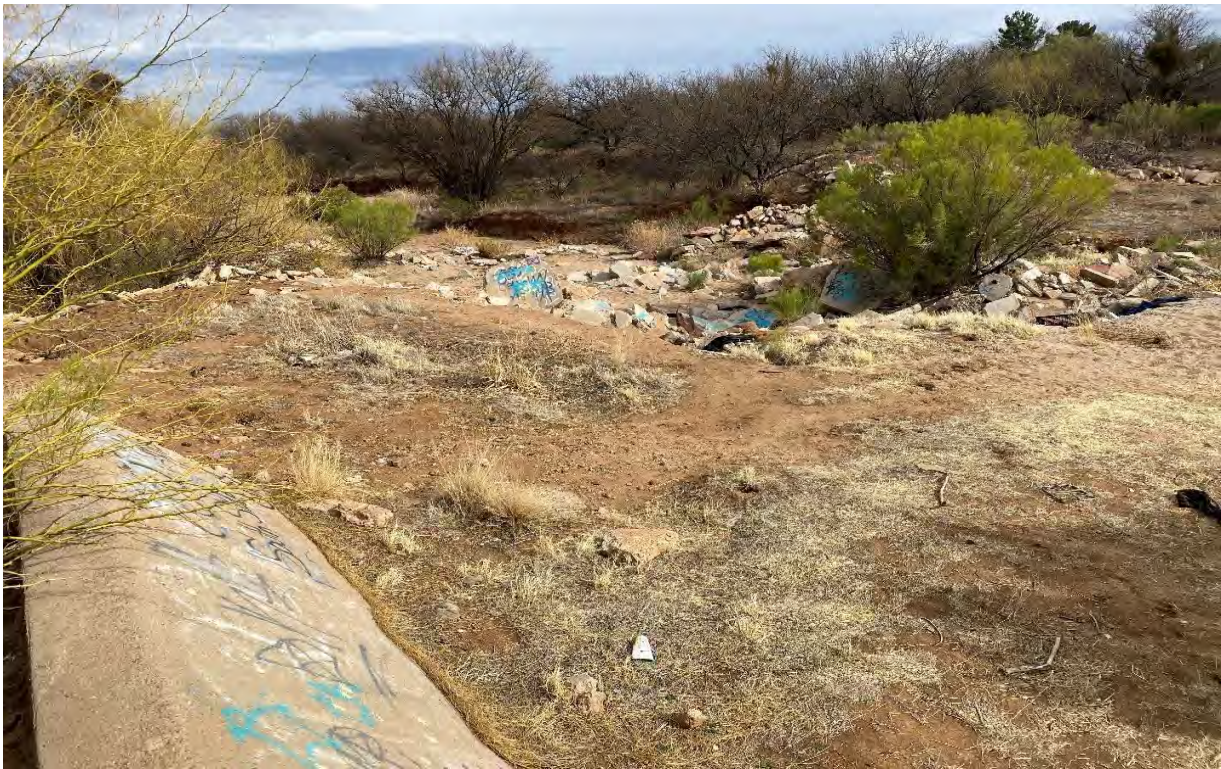
Figure 4.5.1 - Coyote Wash Headcut at Sewer Line Crossing 1940-ft downstream of Foothills Drive
