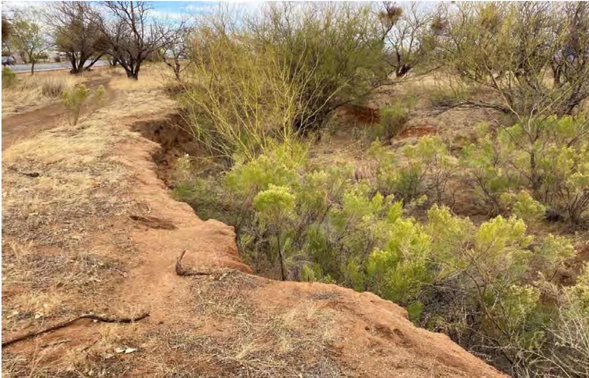
Figure 4.6.2 - Woodcutters Wash Headcut Downstream of Grade Control near 7 th Street/Savannah Drive Intersection
