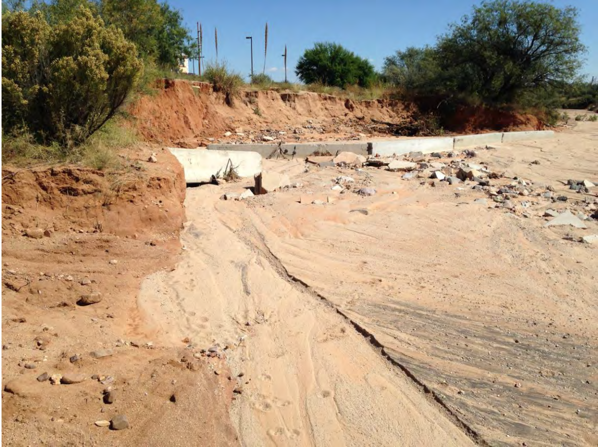
Figure 5.1.3 - Charleston Wash Bank Erosion at Port Royale Apartments
