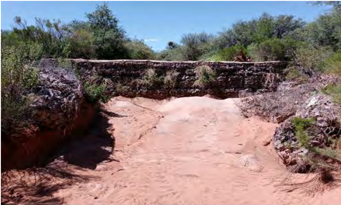
Figure 4.8.2 - Charleston Wash at Sewer Line crossing about 860-feet west of Avenida Escuela
