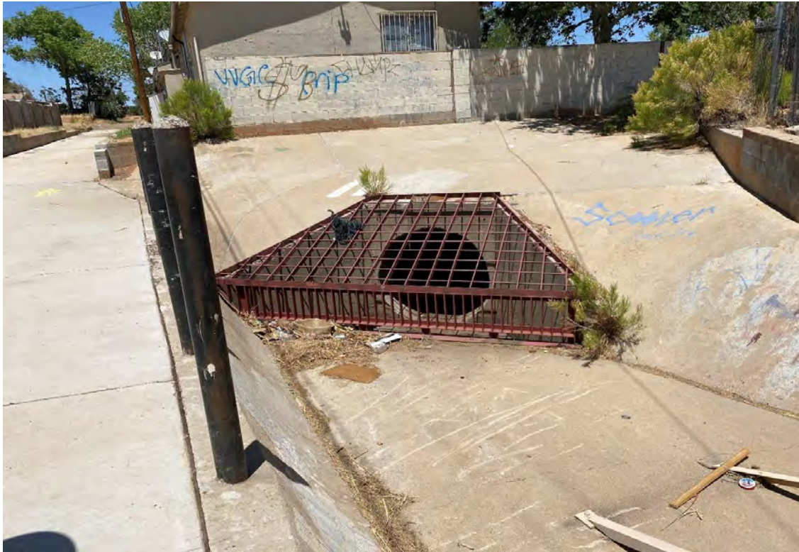
Figure 9.5 - Inlet to 66-Inch Storm Drain Connecting Fab Ave Drainageway to Vista Village Drainageway
