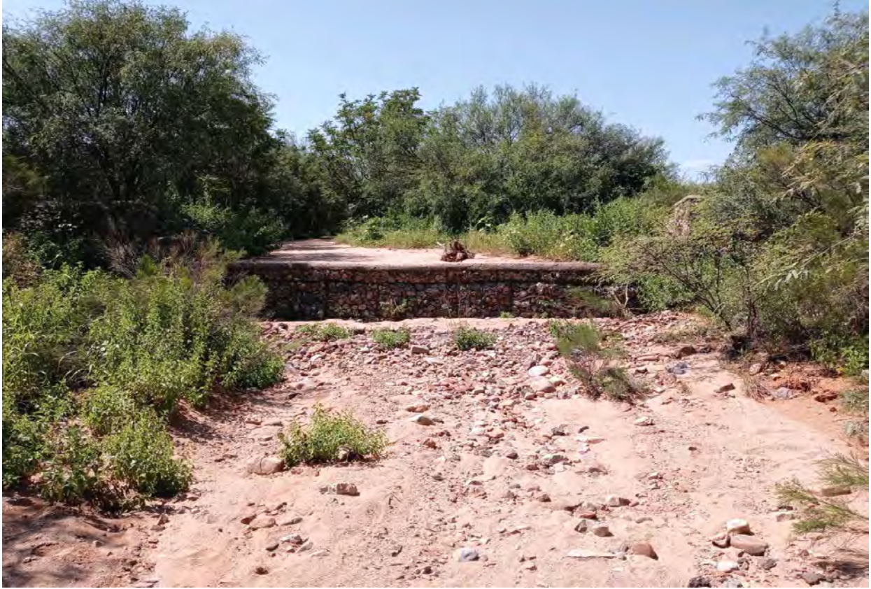
Figure 4.4.2 – Kings Manor Wash Grade Control located about 150-feet Upstream (south) of SR-90
