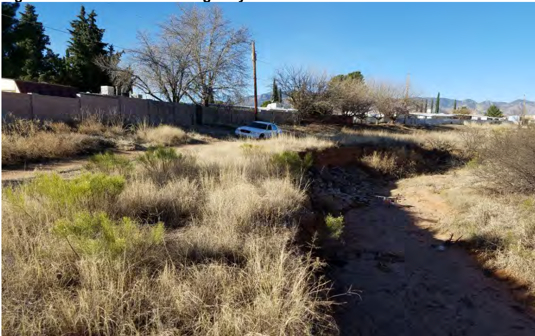
Figure 5.1.2 - 3 rd Street Drainageway Bank Erosion near Sewer Line
