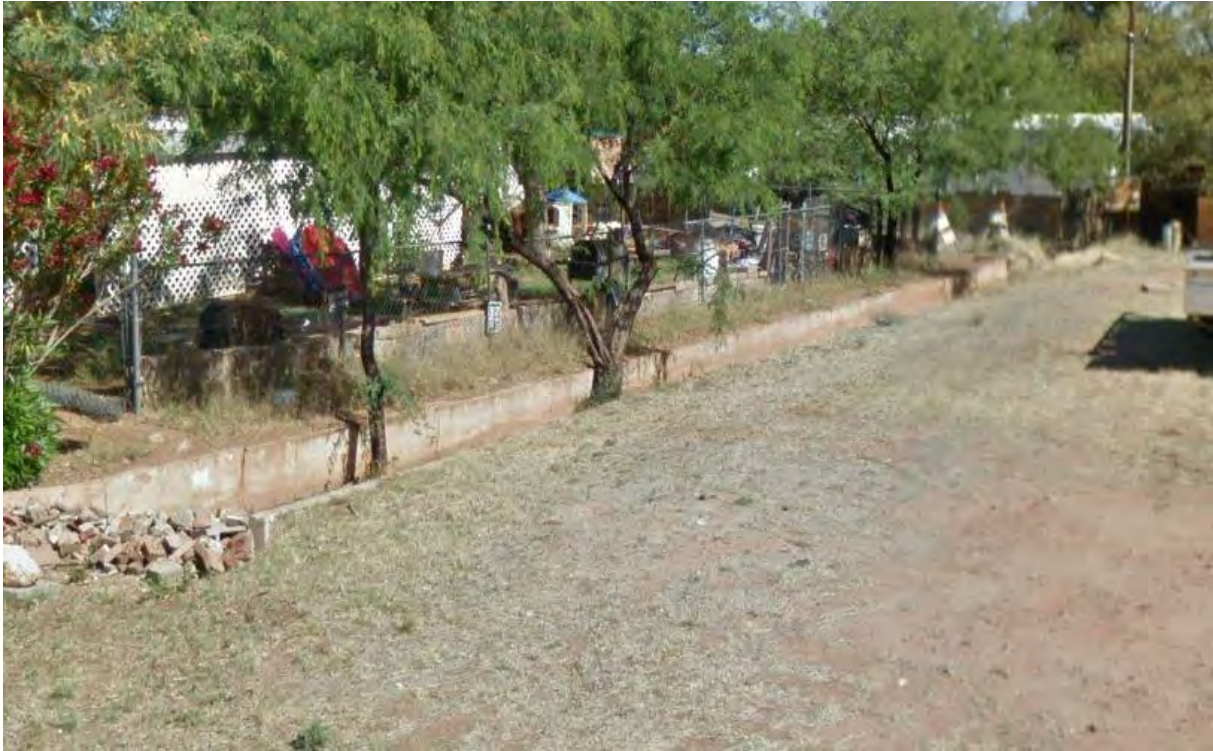
Figure 4.1.3 - Jennifer Ln –Sulger Subdivision Drainage Ditch between residential lots
